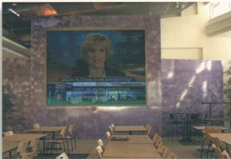
A 4x4 video wall was installed in the Cafetorium to fill an existing hole
